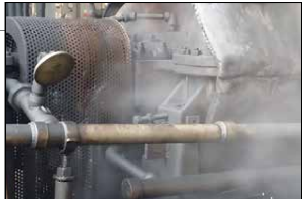
Steam leakage on process steam turbines increases steam costs and leads to lower efficiency and steam turbine performance.
