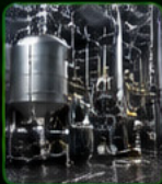
Plants, Tanks & Pipelines
