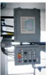
Digital Control Panel
